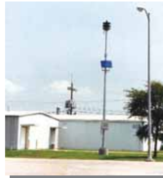
Whelen siren with Solar Regulator in the field.
